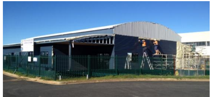
Professionals Syd and Daniel sheeting the southern wall after Aero Club volunteers installed insulation
